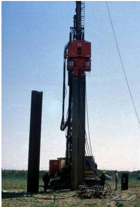
Fig. 9: Trials in the rocky area (driven sheet pile on left, vibrated sheet pile on right)
